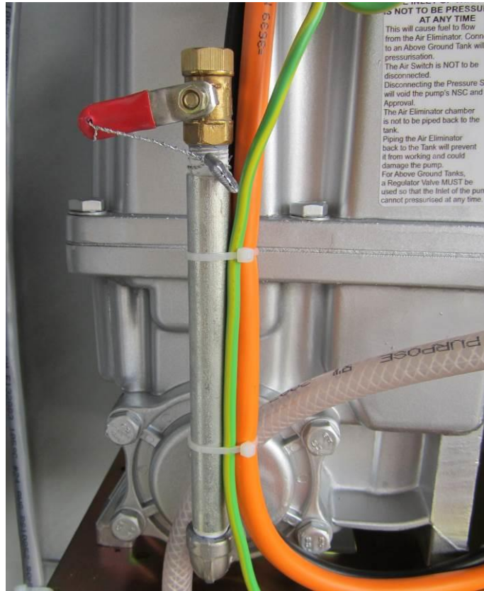
(a) The gas separator test valve
